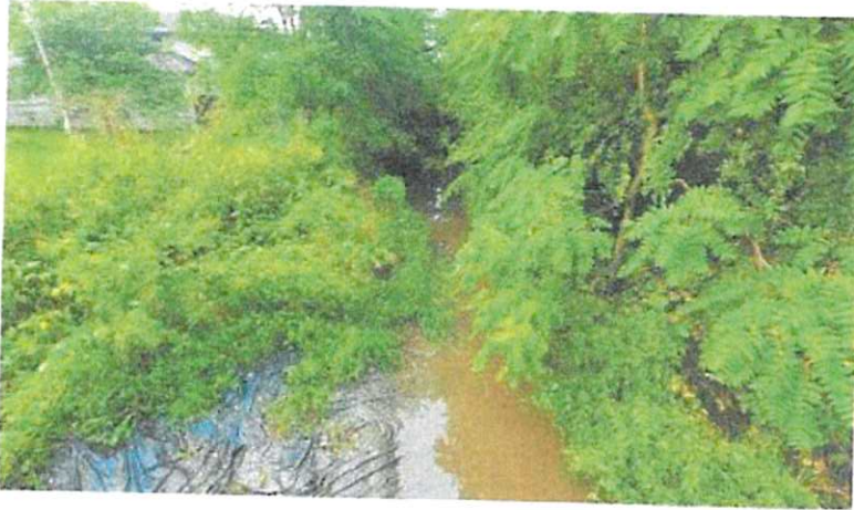
Allen Street facing south. Brush shade hindering grass growth on banks, bare ground underneath allowed to erode during high water and normal rain fall, deposited downstream.
