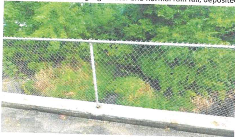
Allen St facing north same issue as above, sediment blocking east duct.
