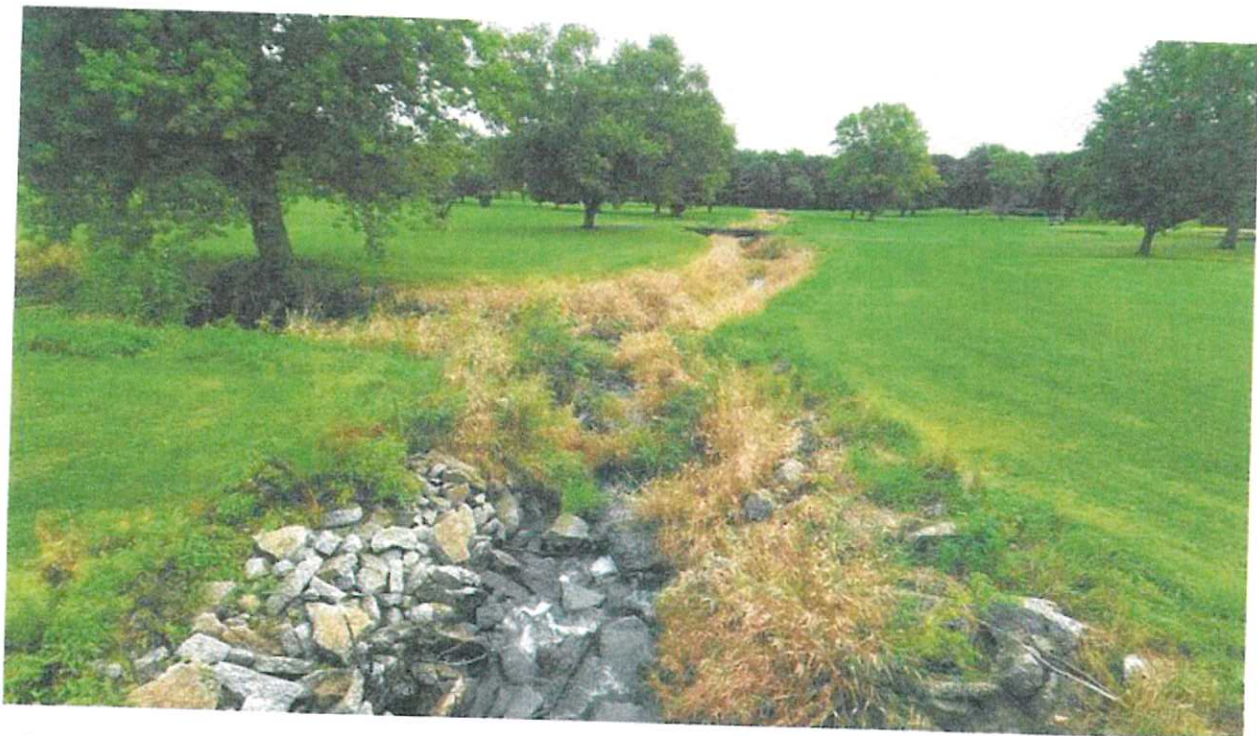
Initial Restriction facing east, Rip Rap impeding water flow causing water to stall and deposit sediment over time.
