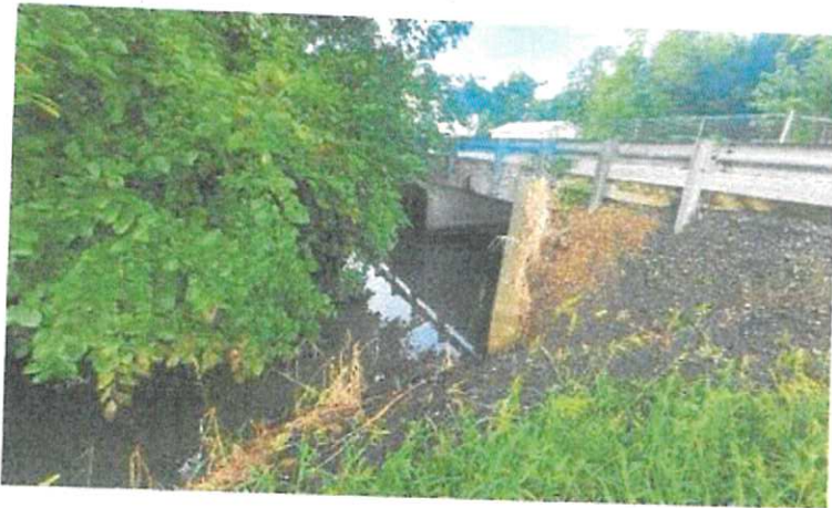
East side of Main Street bridge, Water pooling present.
