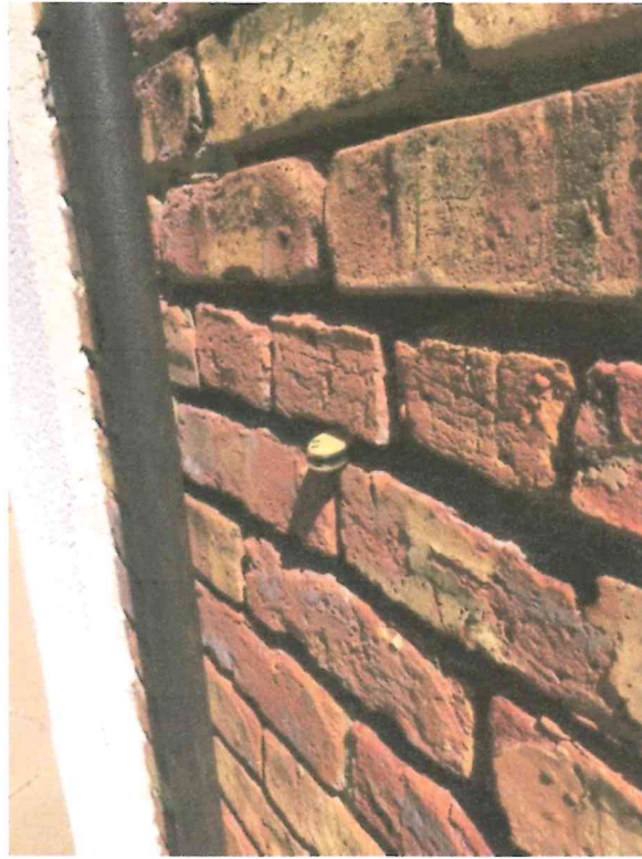
Photograph No. 9 - showing depth of mortar deterioration at location of Photograph No. 8
