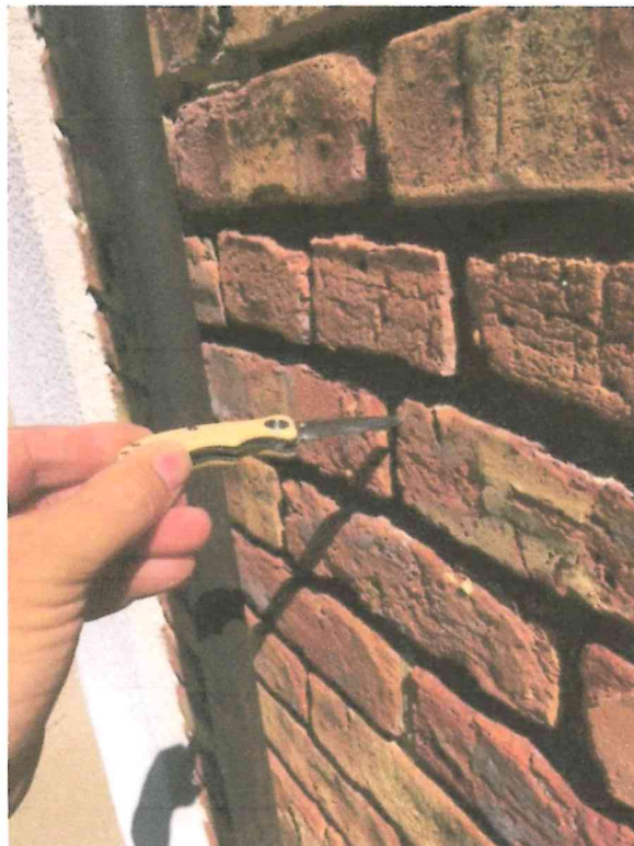
Photograph No. 8 - showing length of deteriorated mortar
