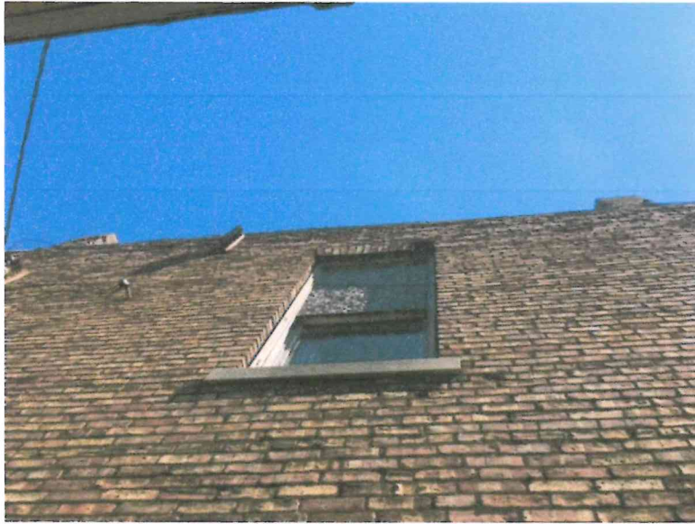
Photograph No. 7 - window above Photograph No. 6 showing missing brick
